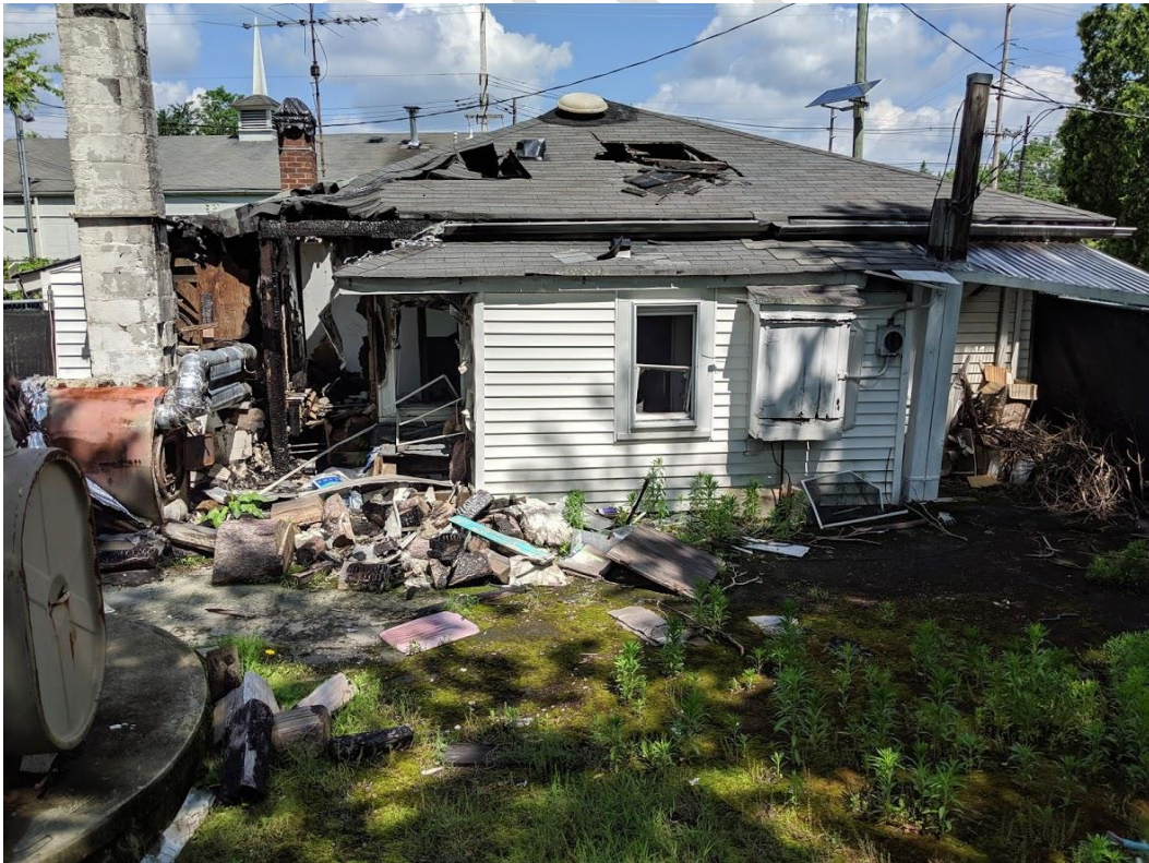
Photograph 37: Block 39 Lot 5 Southerly Side Façade, Showing Fire Damage (photo taken from Lot 7)
