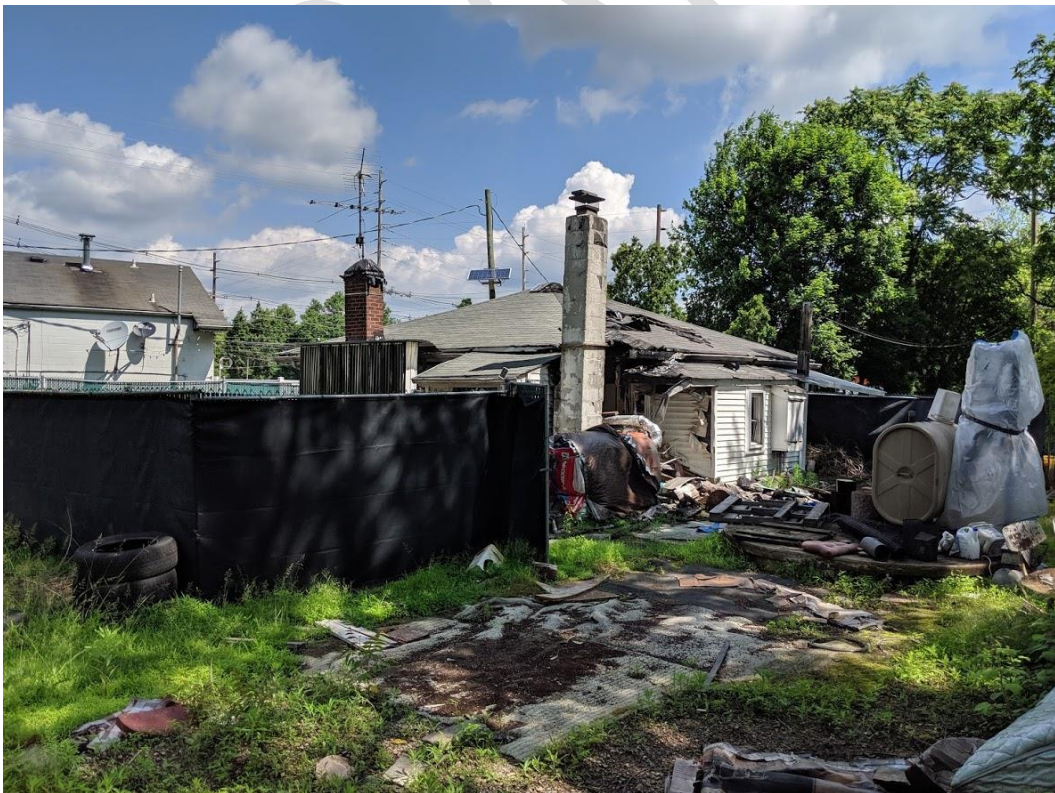
Photograph 39: Block 39 Lot 5 Rear Facade and Rear Yard, Showing Fire Damage (photo taken from Lot 7)
