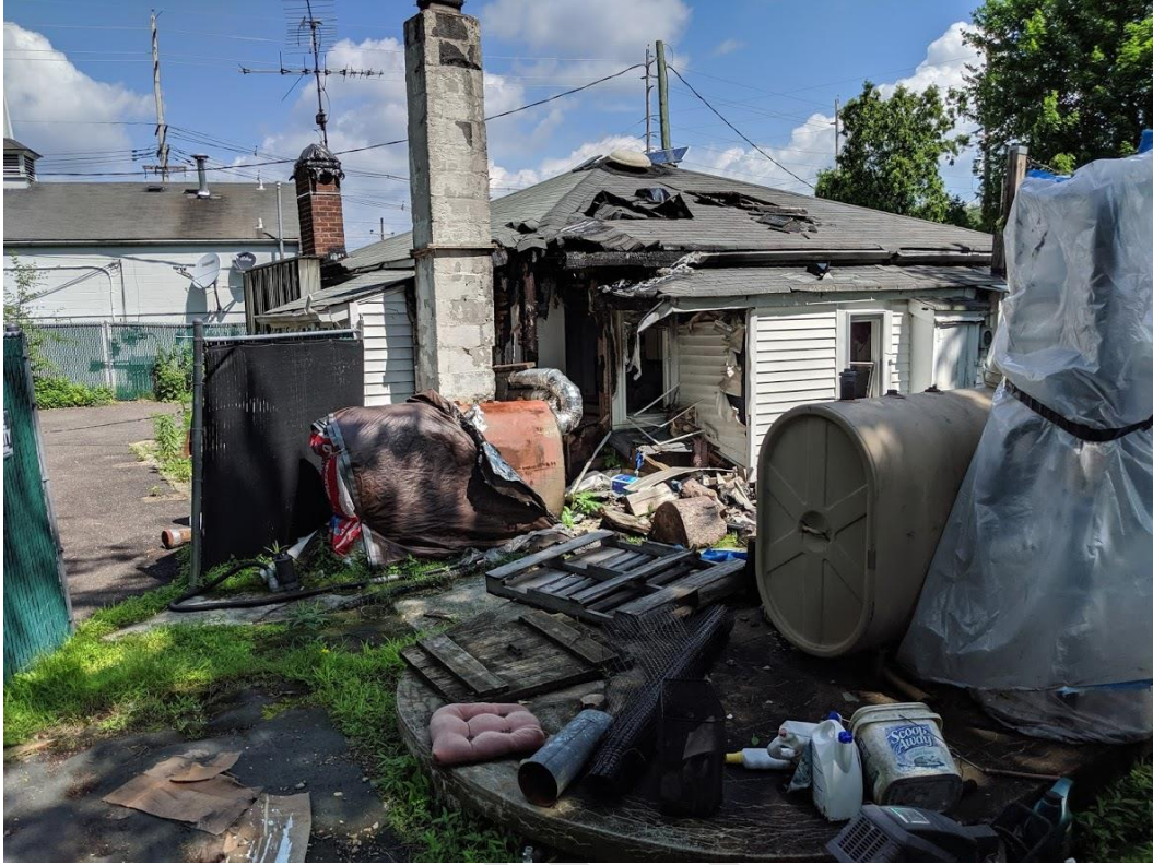
Photograph 38: Block 39 Lot 5 Southerly Side Façade, Showing Fire Damage (photo taken from Lot 7)
