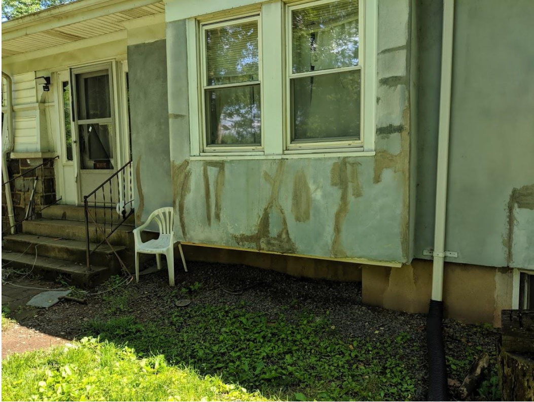
Photograph 24: Block 39 Lot 4 Southwesterly Side Façade of Building (showing patchwork of cracks)
