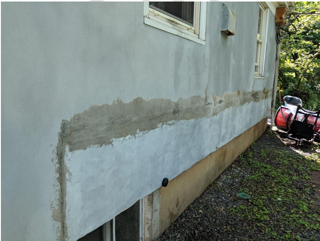
Photograph 25: Block 39 Lot 4 Southwesterly Side Façade of Building (showing patchwork of cracks)
