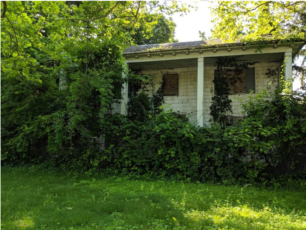
Photograph 4: Block 38 Lot 2 Front Facade of Abandoned Dwelling
